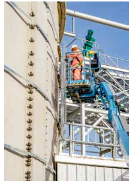
The cladding has not been installed yet, ongoing work on one of the digesters at Mepal III.
