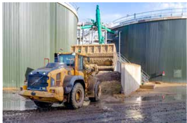
Constantly in motion: The wheel loader feeding the plant with pretreated straw.
