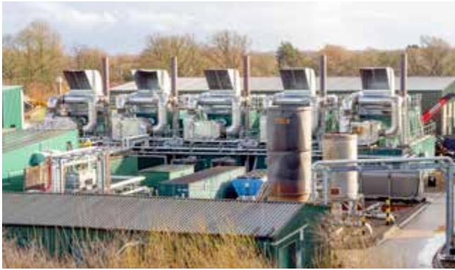
Only Mepal I generates electrical power via generators.
