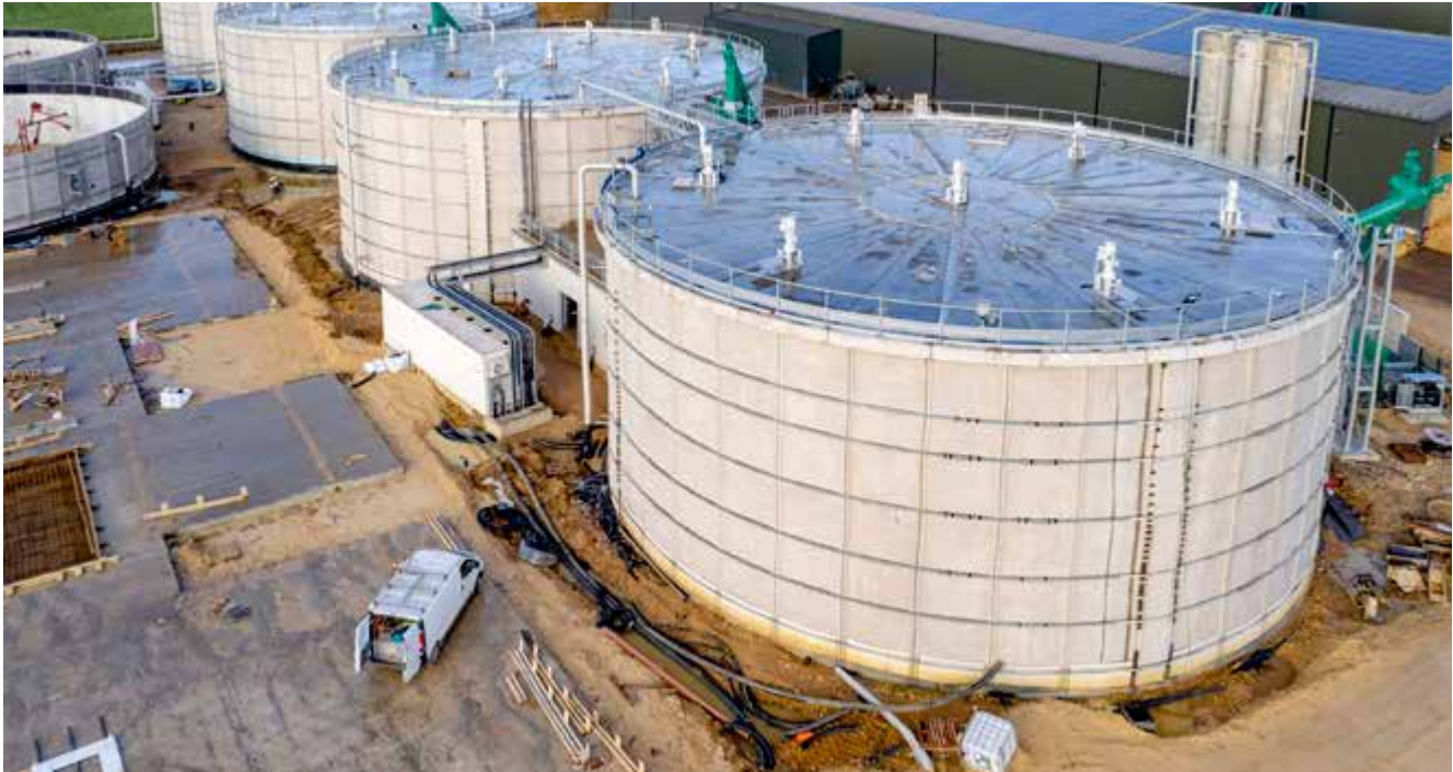
Still in shell construction: The concrete roofs of the digesters at Mepal III are clearly visible.
